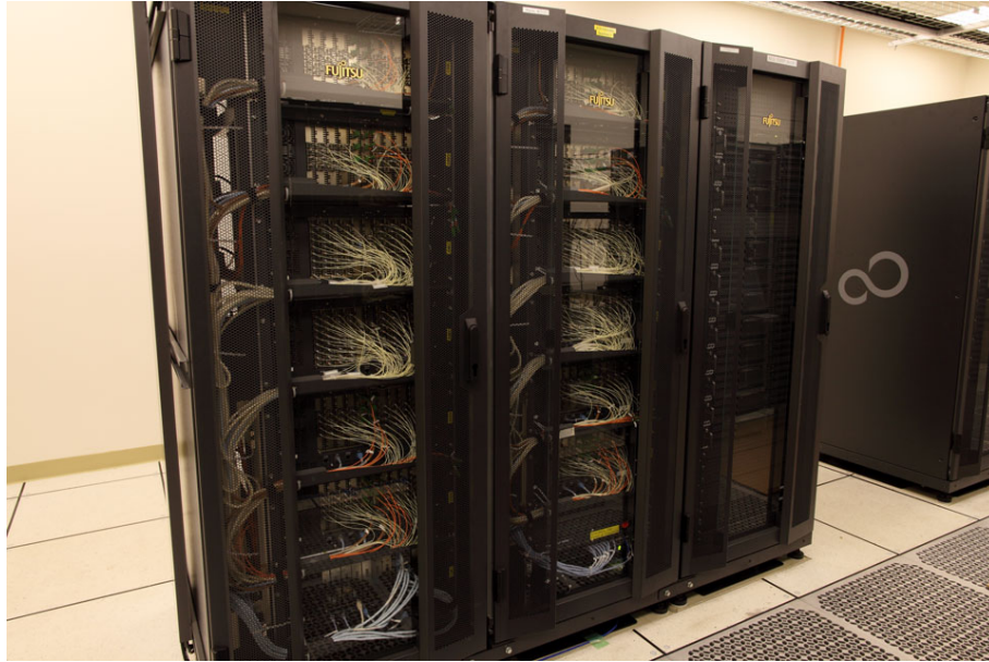
Figure 5.4: Two quadrants of the ALMA Compact Array (ACA) correlator installed in the ACA correlator room. Credit : ALMA (ESO/NAOJ/NRAO), S. Okumura
